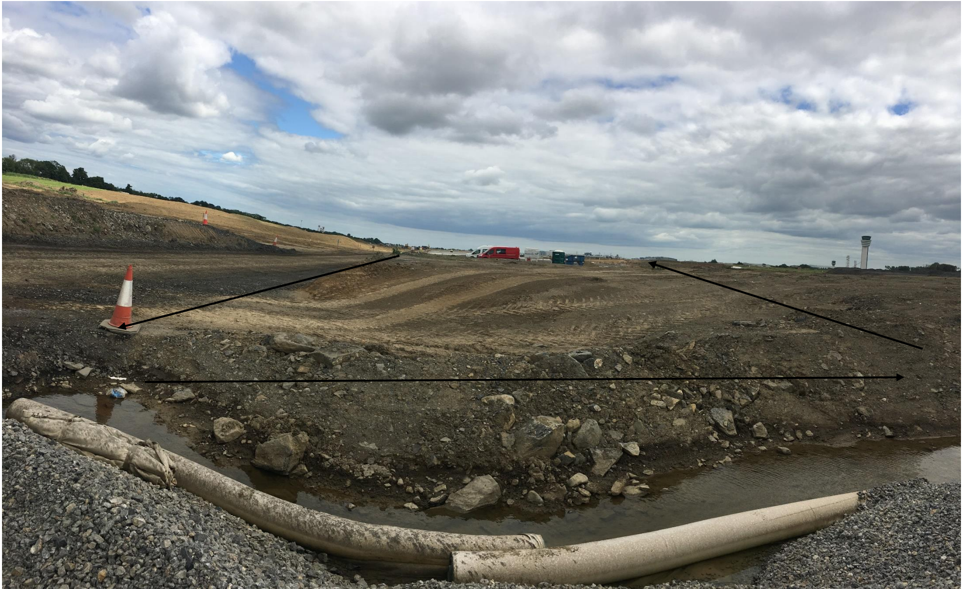
Figure 2: West facing. Approximate depiction of extent of runway footprint - north section of APEC 5
