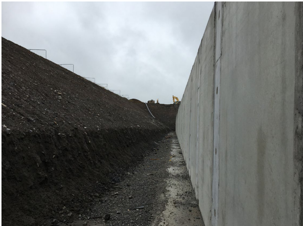
Figure 2-3: Dublin Boulder Clay Structure Below and to the South Side of Tank PWHT
