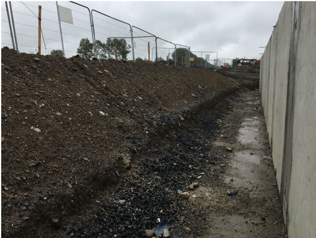
Figure 2-2: Dublin Boulder Clay Structure Below and to the North Side of Tank R2
